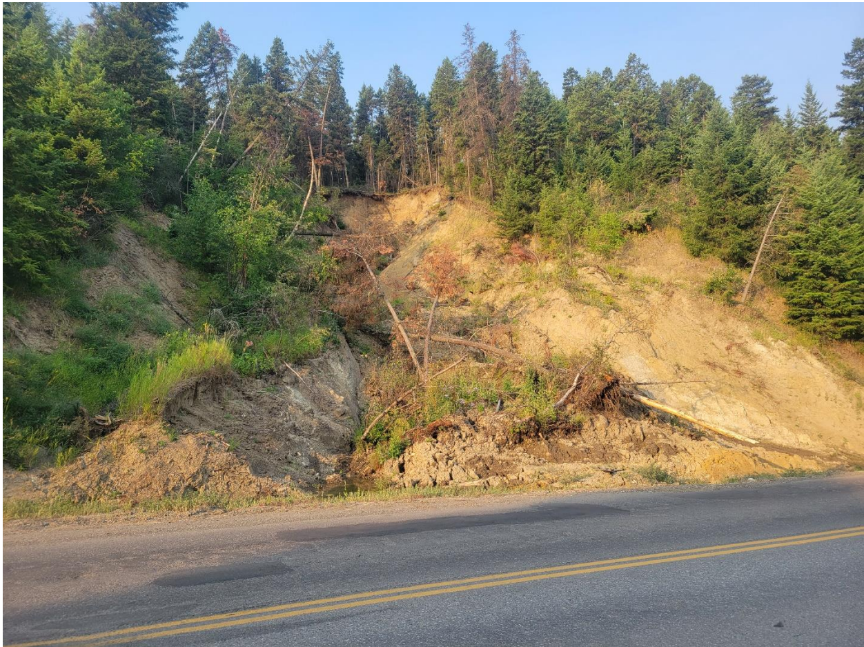
Figure 14. A Landslide on Dog Creek Road, Southwest of Williams Lake.
