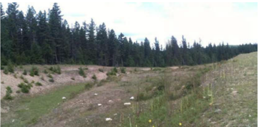
Photo 8. Ditching and capped fill slopes along the western boundary of the Landfill.
