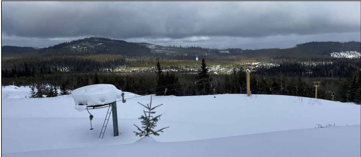
Existing Platter Lift
