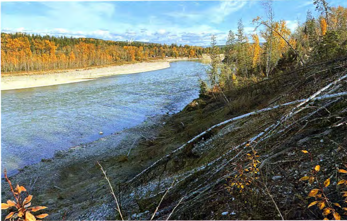
Photo 1. Top-down view of the proposed riprap revetment location at the toe of the North Fraser slide looking downstream. Photo taken on October 11, 2023.
